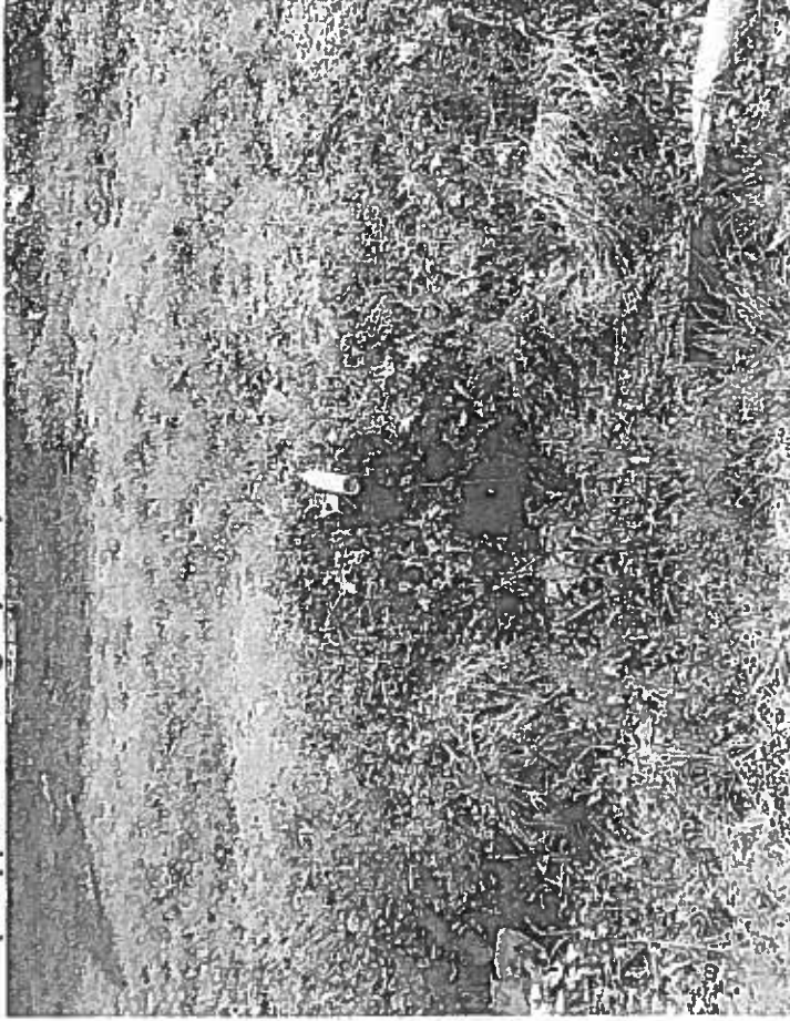
Above pictures shows unapproved sewage discharge line from old cesspool to ditch.
